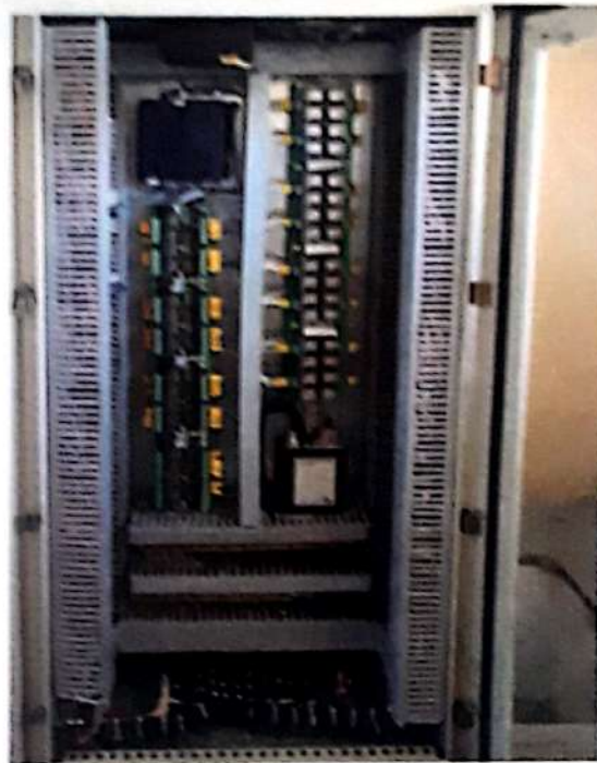
Panel SCADA & DC
