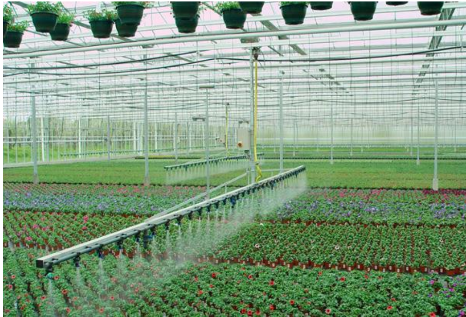
Figura 1.4. Irrispray-Fixed- I Watering Irrigation System
